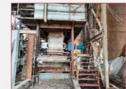
Relocation of AF Equipment's
