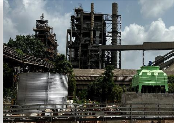
DM Tank and Auxiliary Cooling Tower
